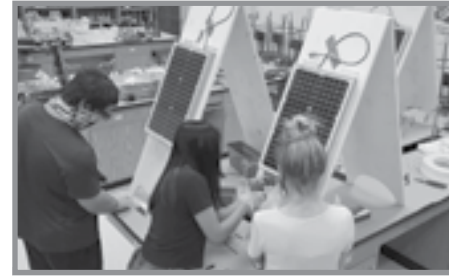
Trenton Liner, Claudia Lopez and Courtney Parrish attach solar panels to the A-frames
