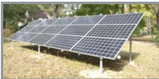
NAPS Members Lynton Land & Judy Lang installed a ground-mounted solar array at their residence in Ophelia a year ago.
